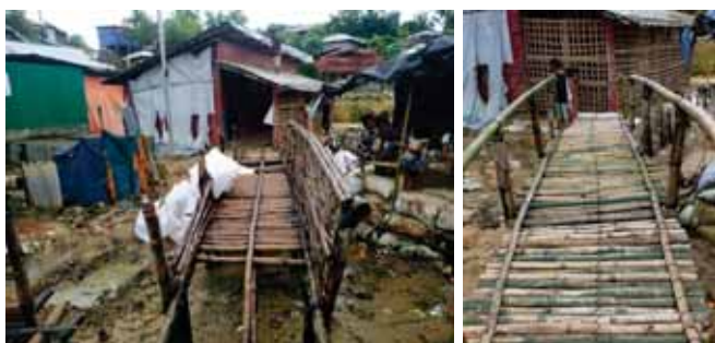
It's a part of LC repair work of Rose LC in Camp-2. Picture: Minar(M&E)
