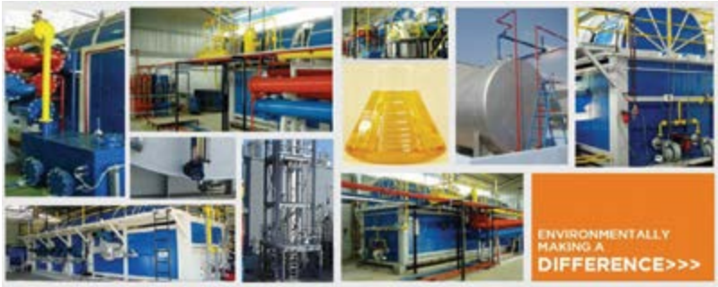
MK Aromatics Limited state of the art "waste plastic to fuel" facility. Source: (www.mkaromatics.com)
