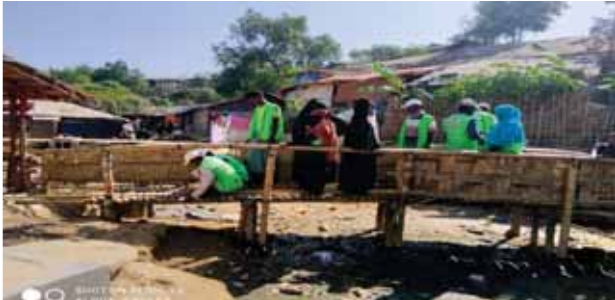
Learning centre comes and out pathway bamboo broken Bridge are repairing. Pic: Alam Badsha (PE)
